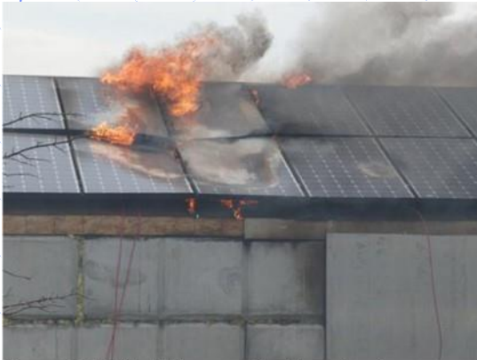
Figure 175 Modules sagging from heat
